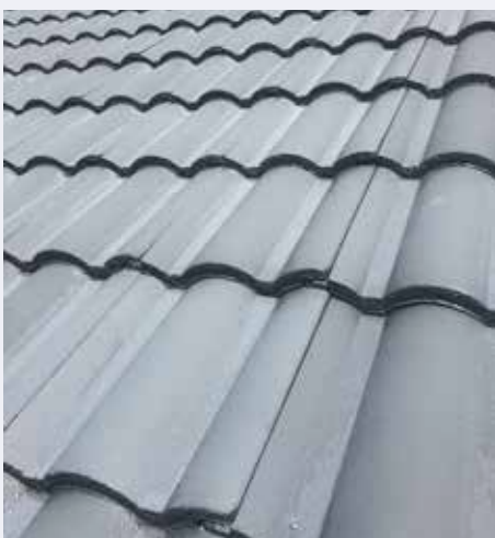
Does your roof appear faded or dull? Environmental fallout such as salt residue, dirt or dust deposits can cause this aesthetic change.
